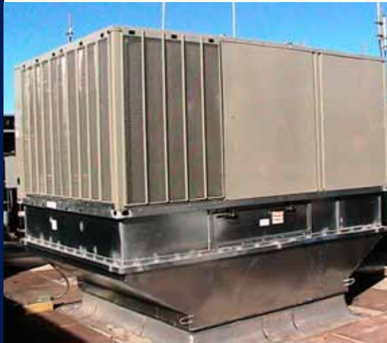
Norman Oklahoma Police Station RTU Change Out
